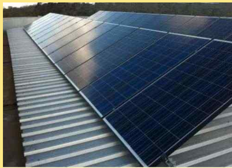
Highfields QLD 7kW system Date of install – September 2014
